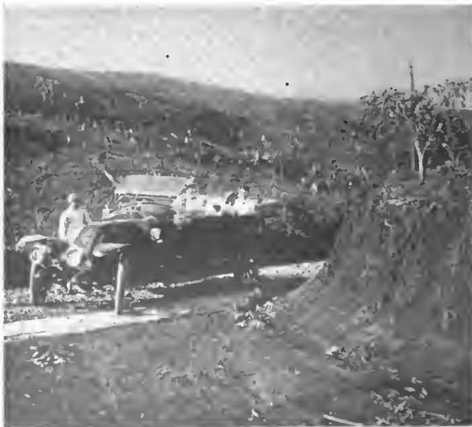
Newly made road in Western Java near Bandoeng. The soil is black, country rolling and the trees cleared off to the ground
